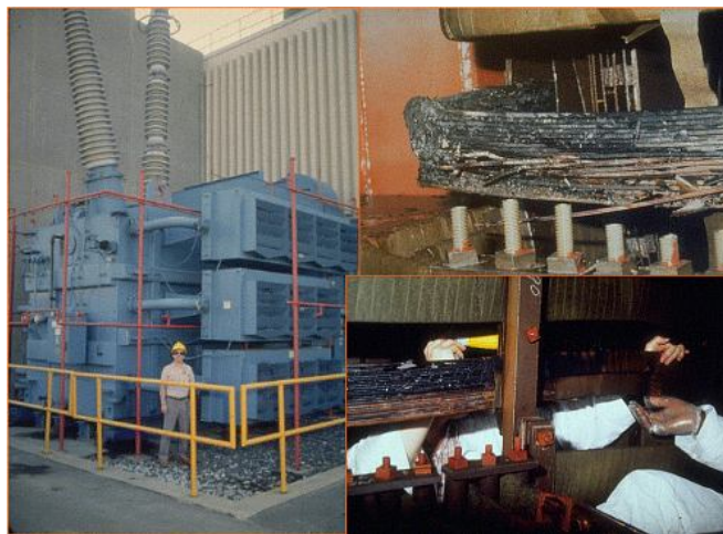
Fig. 4: Melting of transformer windings due to Eddy's current produced by GIC.
